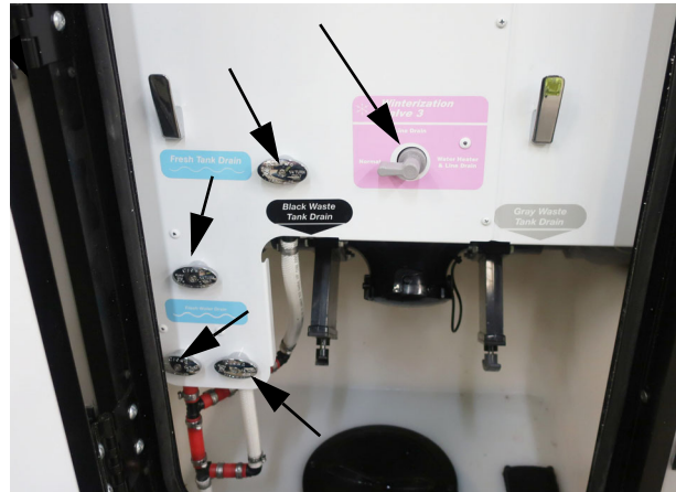
Waterlines and Tank Drain Valves (Shown in the closed position) -Typical View
