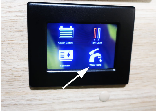
Water Pump Switch on the Systems Monitor Panel. -Typical View
