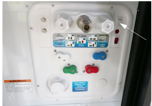
Water pump switch location on Water Center Panel.
