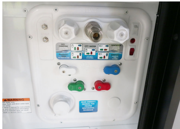
Winterization configuration -Typical View
