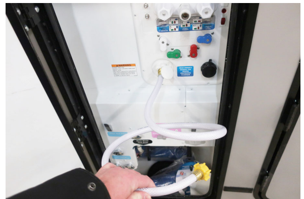
Attach a siphon tube then place it in the chlorine solution container and turn the pump on to begin siphoning contents. (Typical View)
