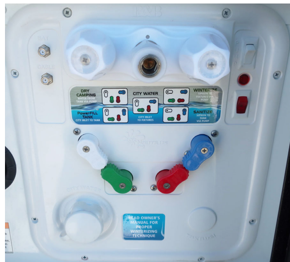
Winterization 3 configuration -Typical View
