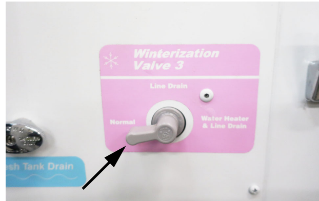
Winterization Valve 3 turned to the “Normal” position. -Typical View
