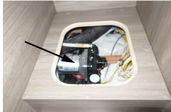
Water Pump (Located inside drivers side bed compartment - remove panel to access) -Typical View
