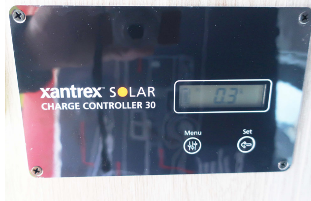
Solar Charge Controller (Located near the monitor panel) -Typical view
