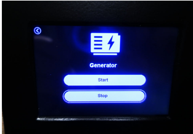
Select the Generator Icon on the main menu to access the Generator start/stop screen. -Typical View
