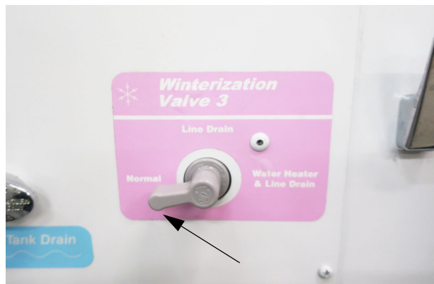
Place the Winterization Valve 3 into the “Normal” position. -Typical View
