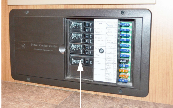
120-Volt Circuit Breakers -Typical View
