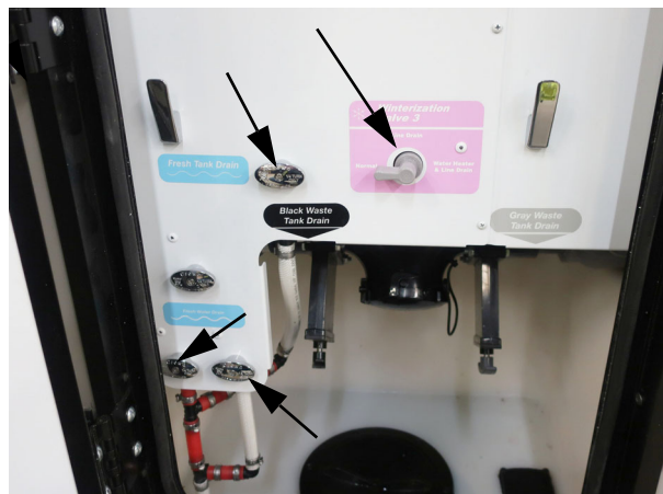
Open the Waterlines and Tank Drain Valves indicated by the arrows. (Shown in the closed position) -Typical View
