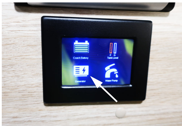
Generator location on the main screen of the Systems Monitor Panel -Typical View
